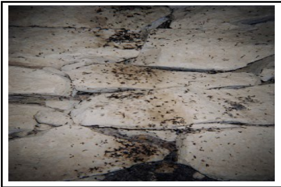
9-1.6 Bat Guano on Riprap
